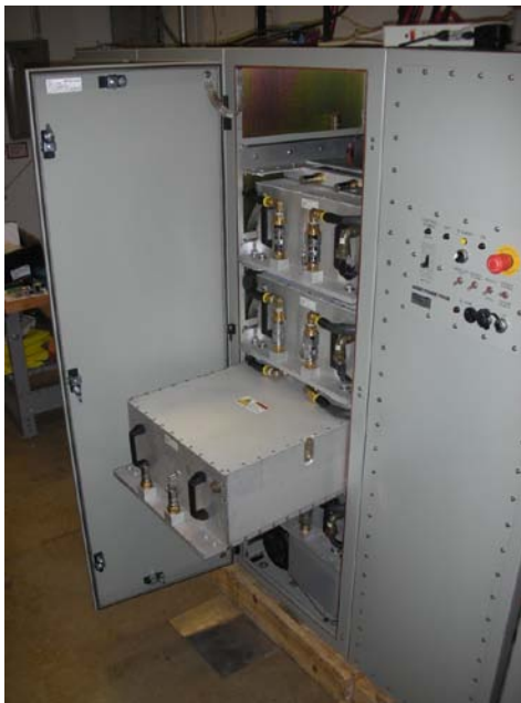
Energy Storage Module Showing Parallel Inverter Modules
