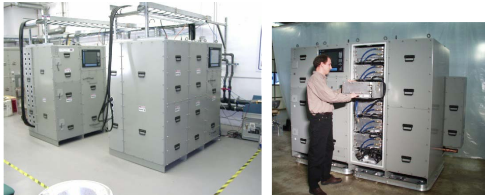
RCT Systems PCMs Installed for Test at the General Atomics Test Site
